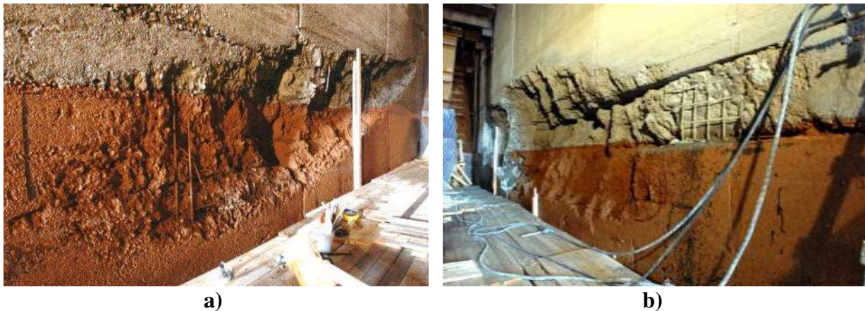
Figure 5: Bureyskaya HPP (Russia). Construction deep spillway, bottom orifice No. 7 (2005): a - right edge (length of concrete damage approximately 12 m); b - left edge (length of concrete damage approximately 18 m).
