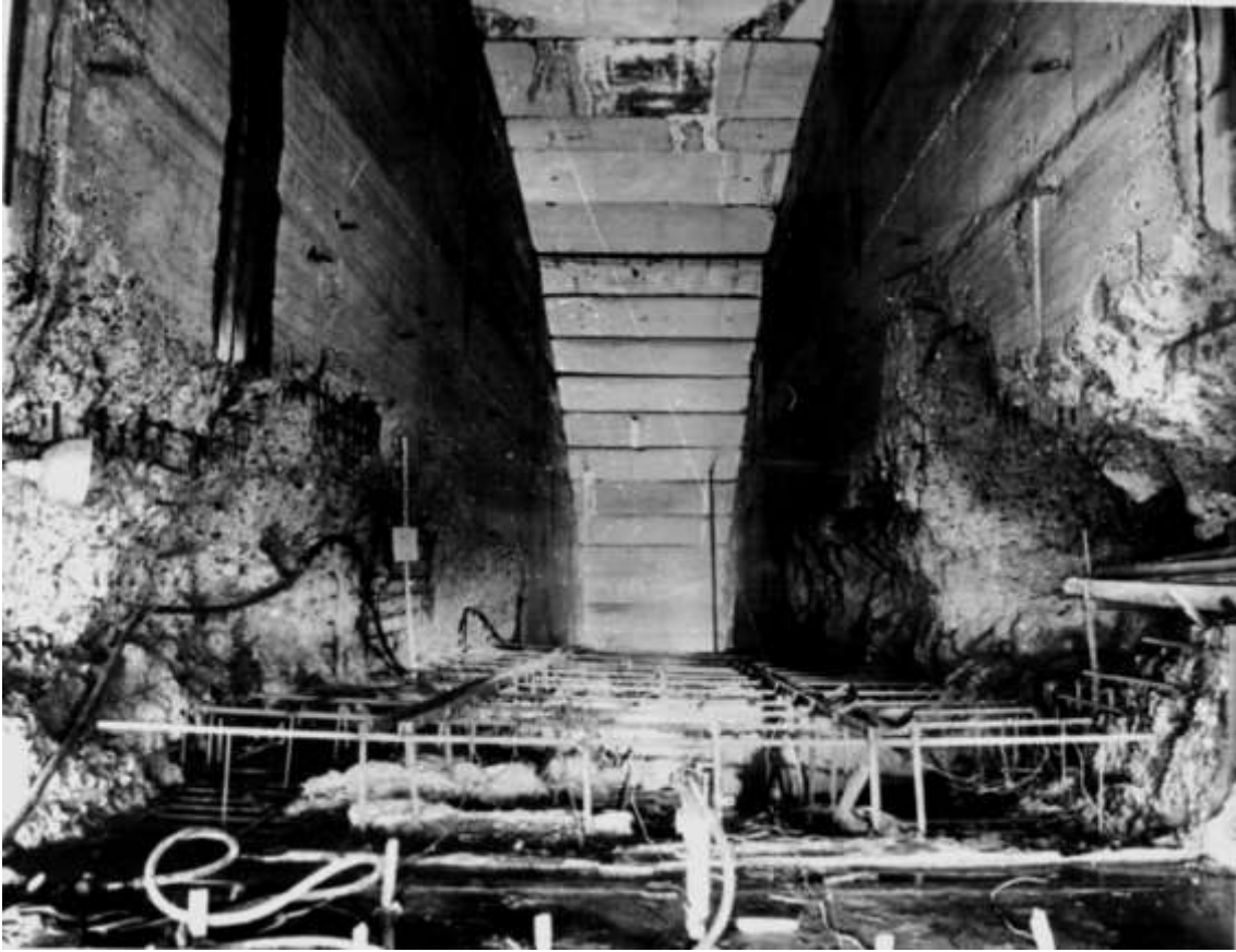
Figure 4: Sayano-Shushenskaya HPP (Russia). Construction spillway of the second tier. Cavitation-induced damages to the floor and sidewalls behind the gate chamber (1980).
