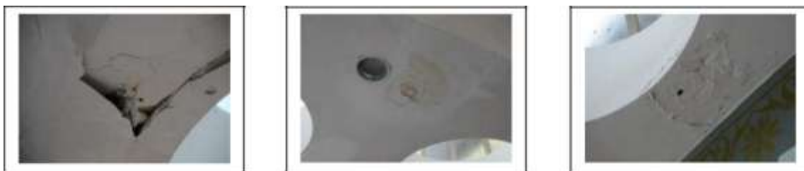
Figure 1: Damage to building ceiling elements, Crystal Mosque, Kuala Terengganu.
