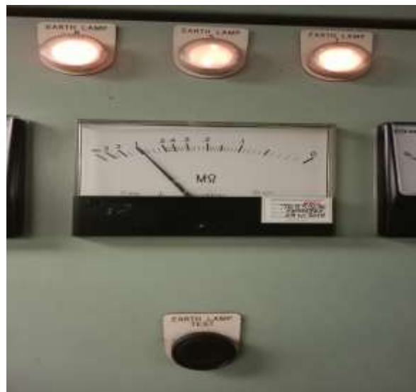
Fig 6: Earth fault indicator on switch board with ohmmeter.
