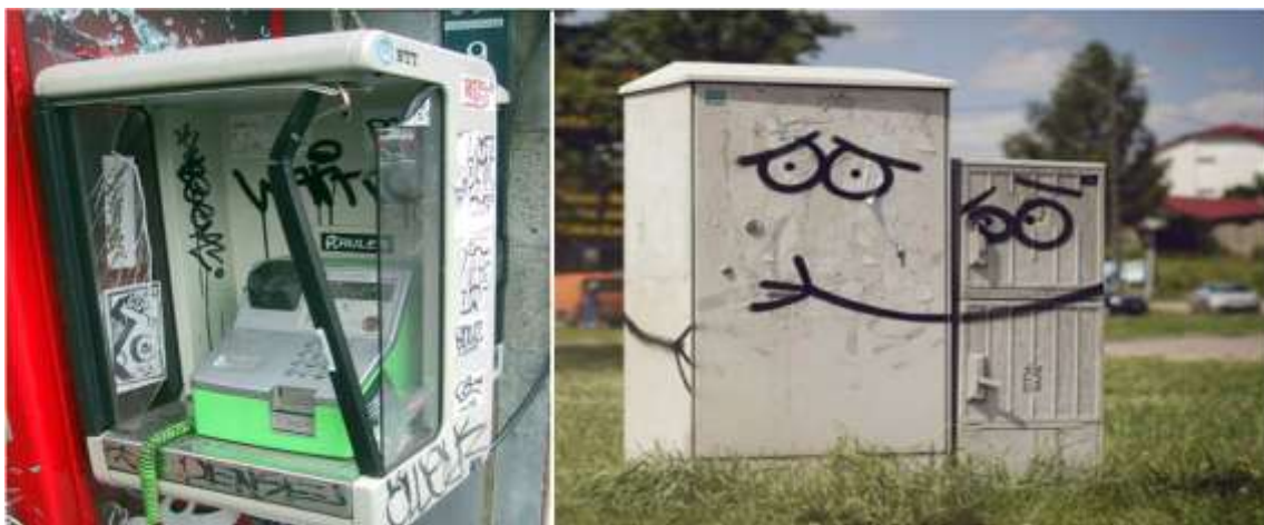
Fig. 2: Examples of vandalism. [12,13]
