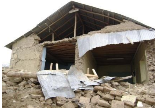
Figure 5: Damaged masonry building in Elazig – Kovacilar used in the study.
