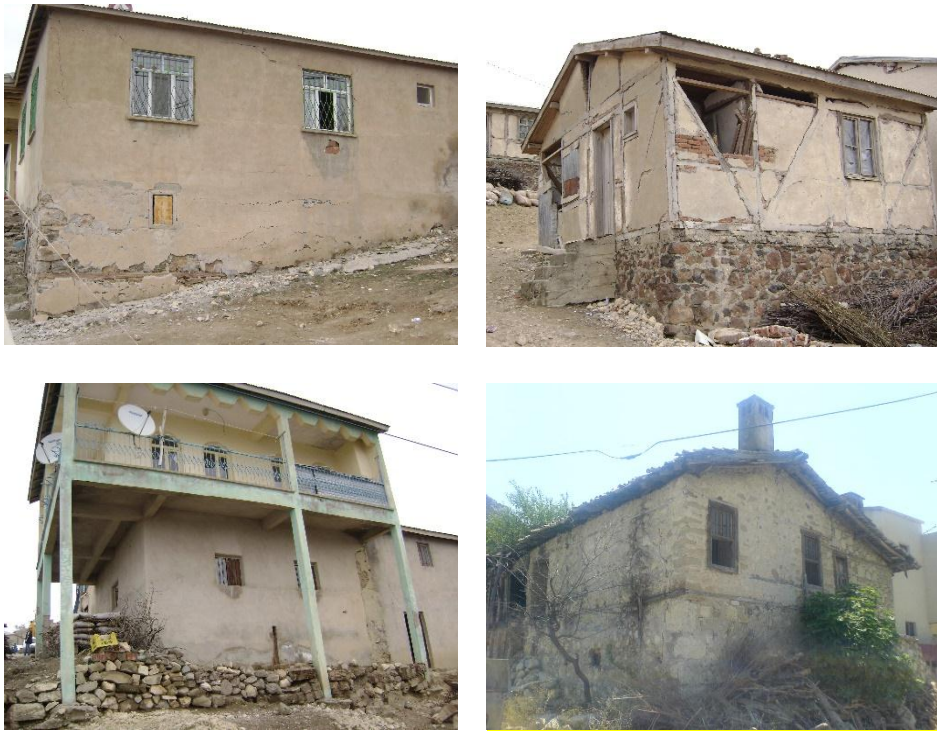
Figure 2: Some examples for Turkish old masonry buildings.
