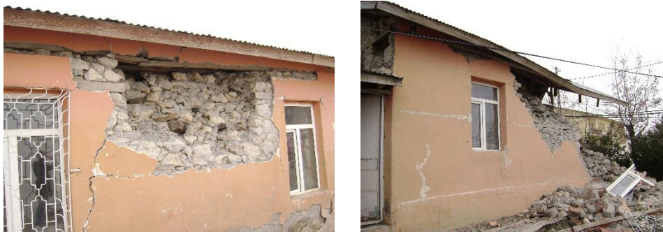
Figure 3: Some examples of masonry failures.
