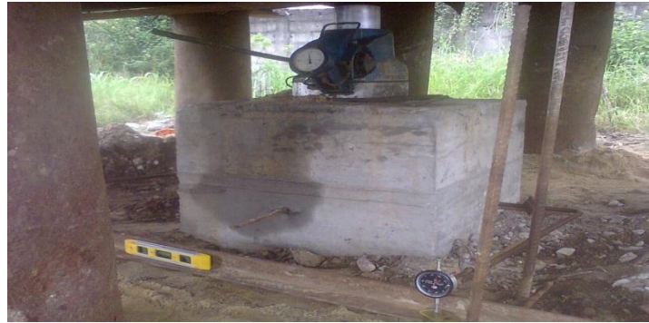
Fig. 2: Failed pile after carrying out testing in Lagos Island.
