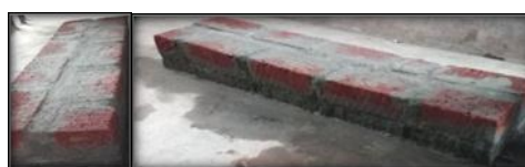
Fig. 2: Finished RCC thin slab and after laying one course of brick masonry.
