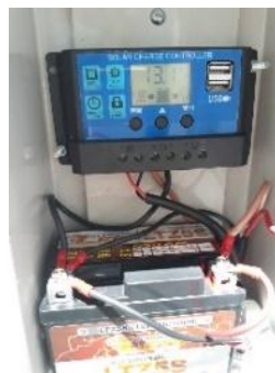
Fig. 7: Control and display system.
