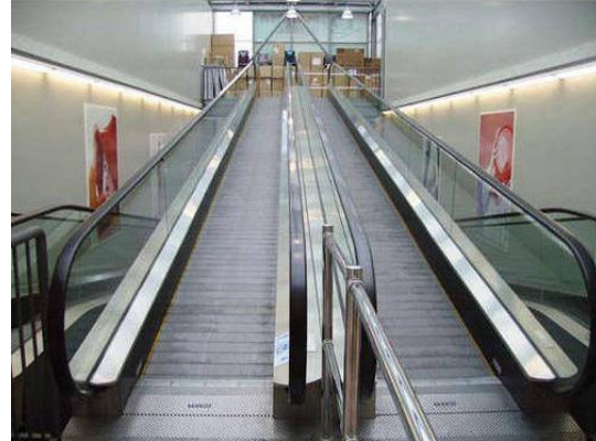
An inclined travellator (linking floors)
