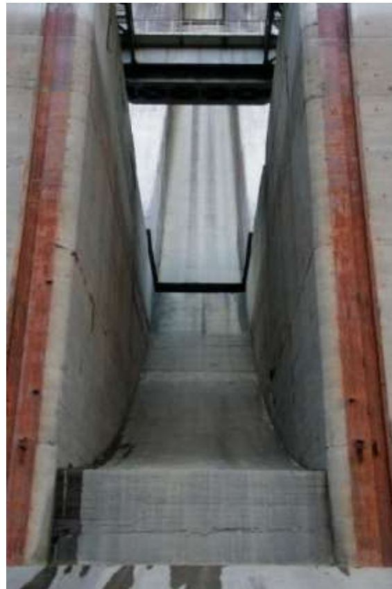
Figure 21: Sayano-Shushenskaya HPP, Russia. Spillway Section 45 after 230 Days of Operation with Flow Velocities Exceeding 55 m/s.
