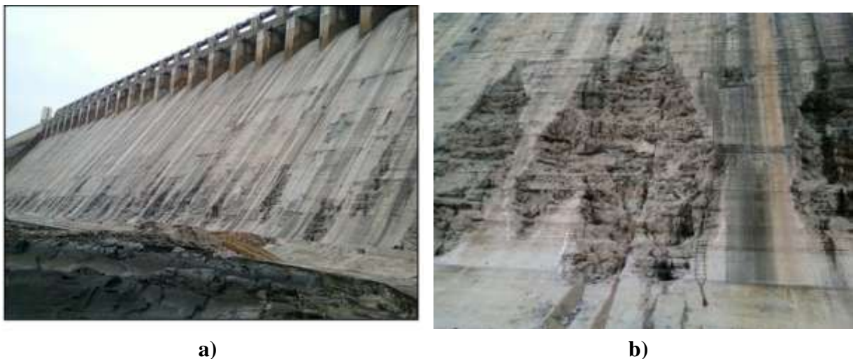
Figure 3: Nagarjuna Sagar Dam (India): a - erosion of spillway during the floods of 2009; b - cavitation damage on dam (Rajasekhar et al., 2014).
