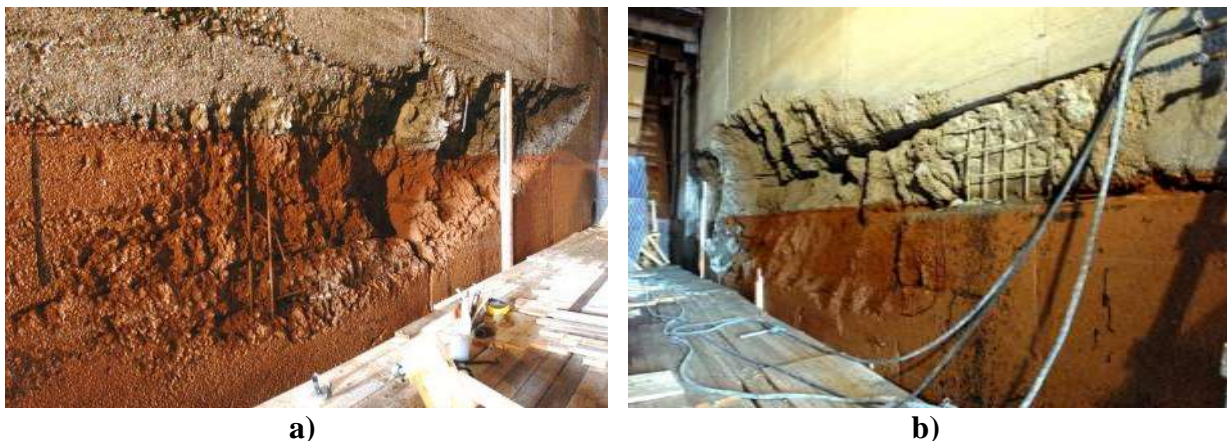
Figure 5: Bureyskaya HPP (Russia). Construction deep spillway, bottom orifice No. 7 (2005): a - right edge (length of concrete damage approximately 12 m); b - left edge (length of concrete damage approximately 18 m).
