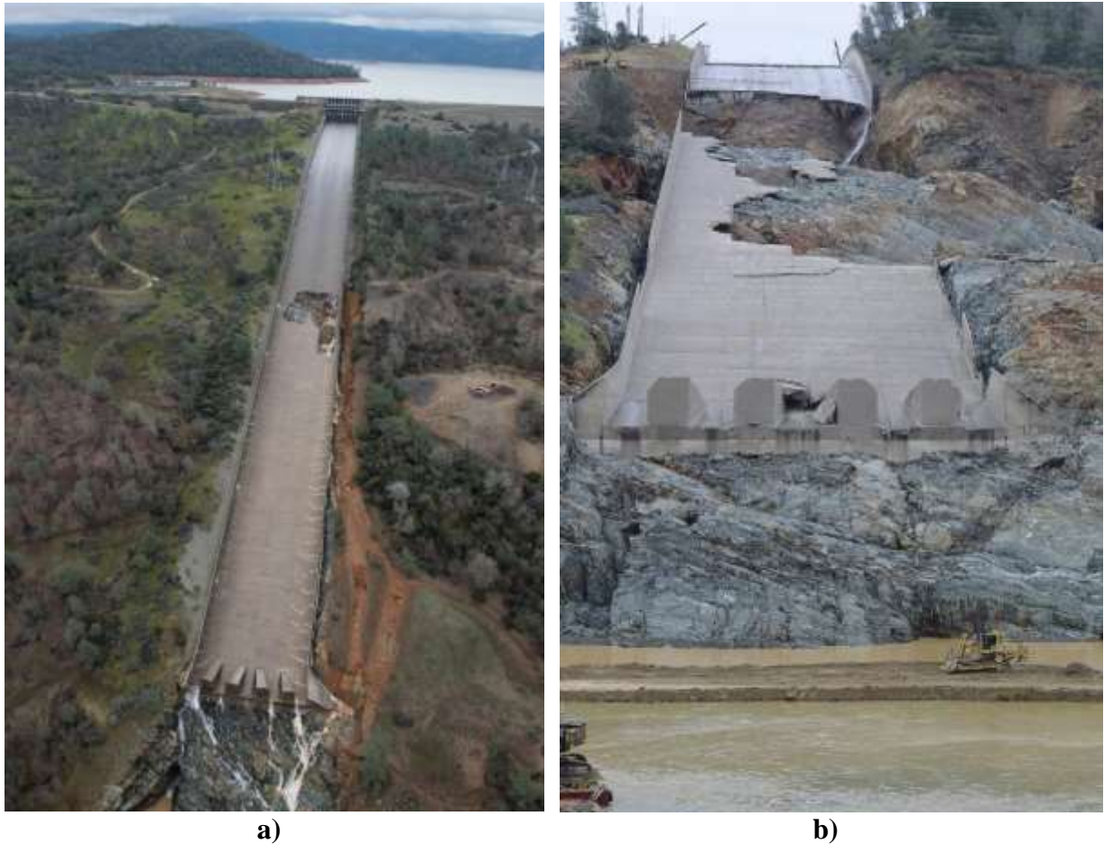
Figure 2: Oroville Dam (USA). Spillway chute damage (Oroville Dam, 2018): a - This initial erosion hole at the service spillway was examined by a climb team on the morning of February 8, 2017; b - Ultimate damage at the service spillway.
