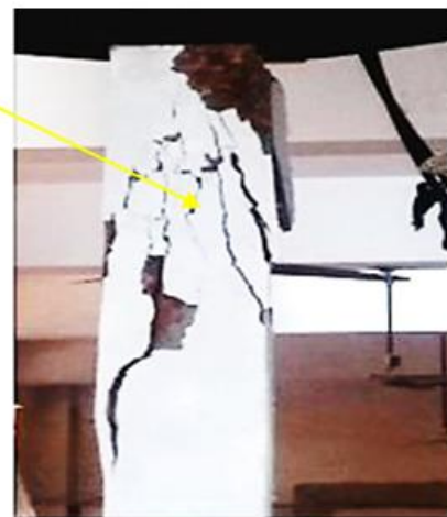
Figure 5 Crushing of the concrete at the Column NC1.
