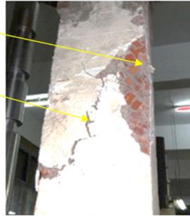
Figure 7 Crushing of the concrete at the Column NS1.
